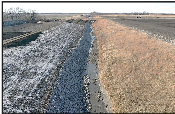
District drone picture of County Ditch 96 Outlet Project facing west from the Red Lake River to Highway 32.
